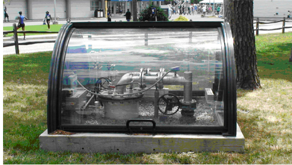
Well pump / Frank Nitti III
