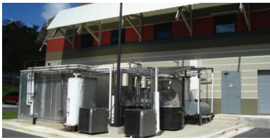
AHU located on Equipment Pad
